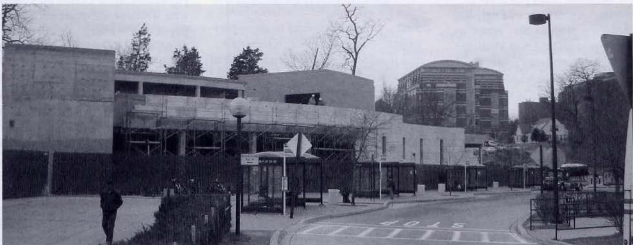
A view from Rockville Pike shows construction of the new two-level Visitor Center, one of three components of the Gateway Project.
