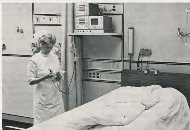
Wall panels contain all equipment for surveillance of individual patients in the newest intensive care units. Each unit has its own power source and suction equipment.
